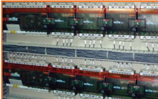
An array of controllers
