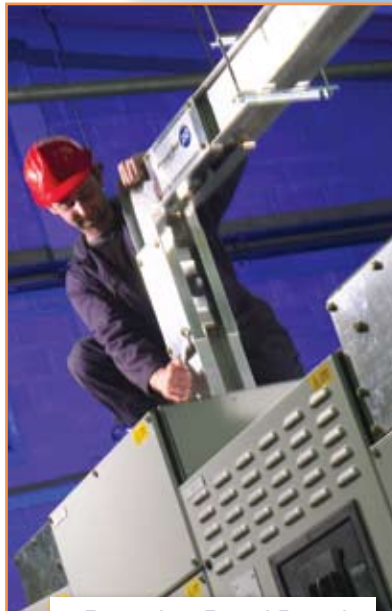
Powerbar Panel Board Connection
